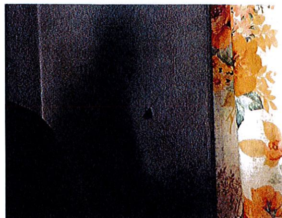
245-1 Bedroom 2 Plaster None Detected
